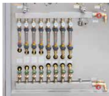
Cooling water distribution
