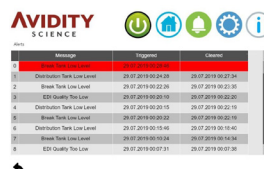
Touch Screen showing alarm interface
