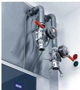
Connection of H2O2 Generator for Moving Heat-Sensitive Materials through Airlocks
